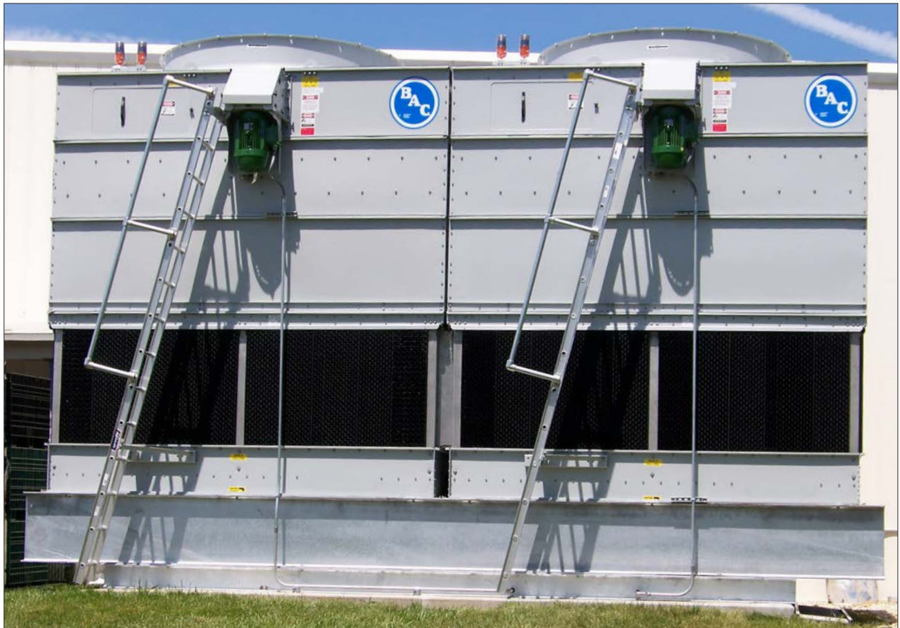
Two-cell PT2 Installation
